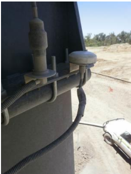
Figure 5: Poor GPS antenna mounting
