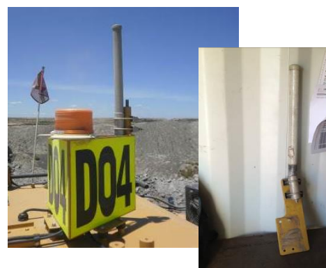
Figure 3: Wi-Fi Antenna damage
